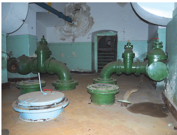
Fig. 9. Toruń – the former Nowe Bielany pumping station: machine room, in the lower left corner the casing of the collecting well, in the background the passage to the chlorination plant (photo by D. Jagiełło, 2024)
