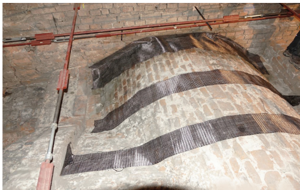
Fig. 3. Vault during installation of carbon mesh composite reinforcement (photo by Ł. Bednarz)
