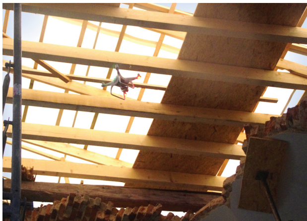
Fig. 1. Visual inspection of a failing vault using a drone (photo by G. Wojciechowska)
