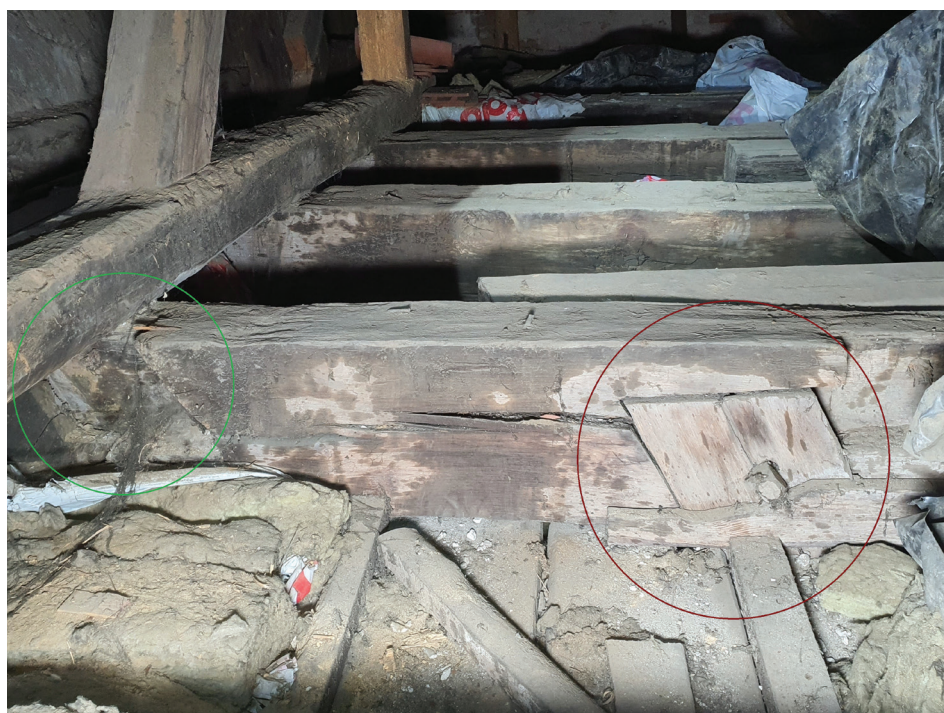
Fig. 7. Church of Our Lady of the Rosary in Byków, the end of the brace connecting with the entablature of the body (red) and the empty mortise after the lap joint of the king strut frame (green) (photo by M. Prarat, 2022)
