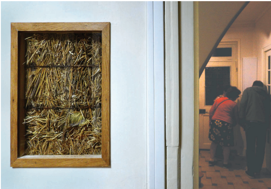
Fig. 5. Interior of the building "Maison Feuilette" in Montargis: in the foreground, the "truth window" providing a glimpse inside the wall, on some century-old straw bales (photo by M. Jagielak, 2015)
