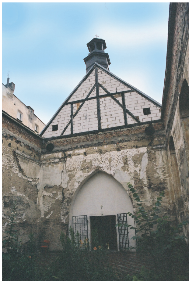
Fig. 5. Zabkowice Śląskie, former Roman Catholic church, view of the ruined nave walls, 2003 (photo by J. Uścińowicz)
